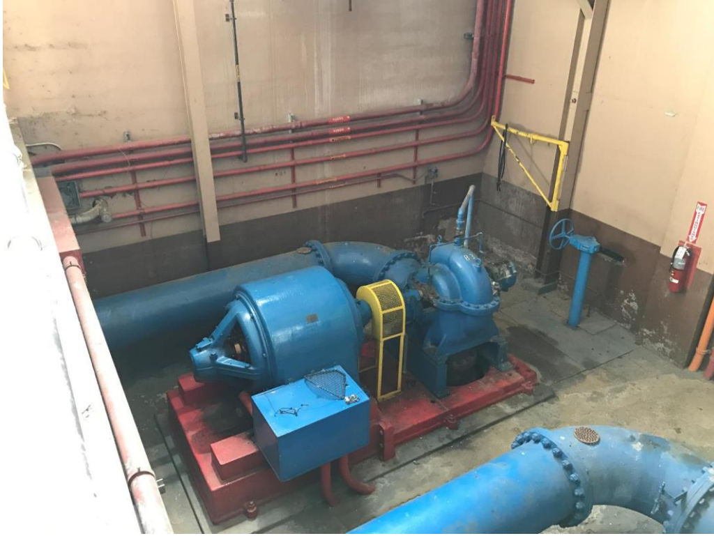
Pump basement looking east.
