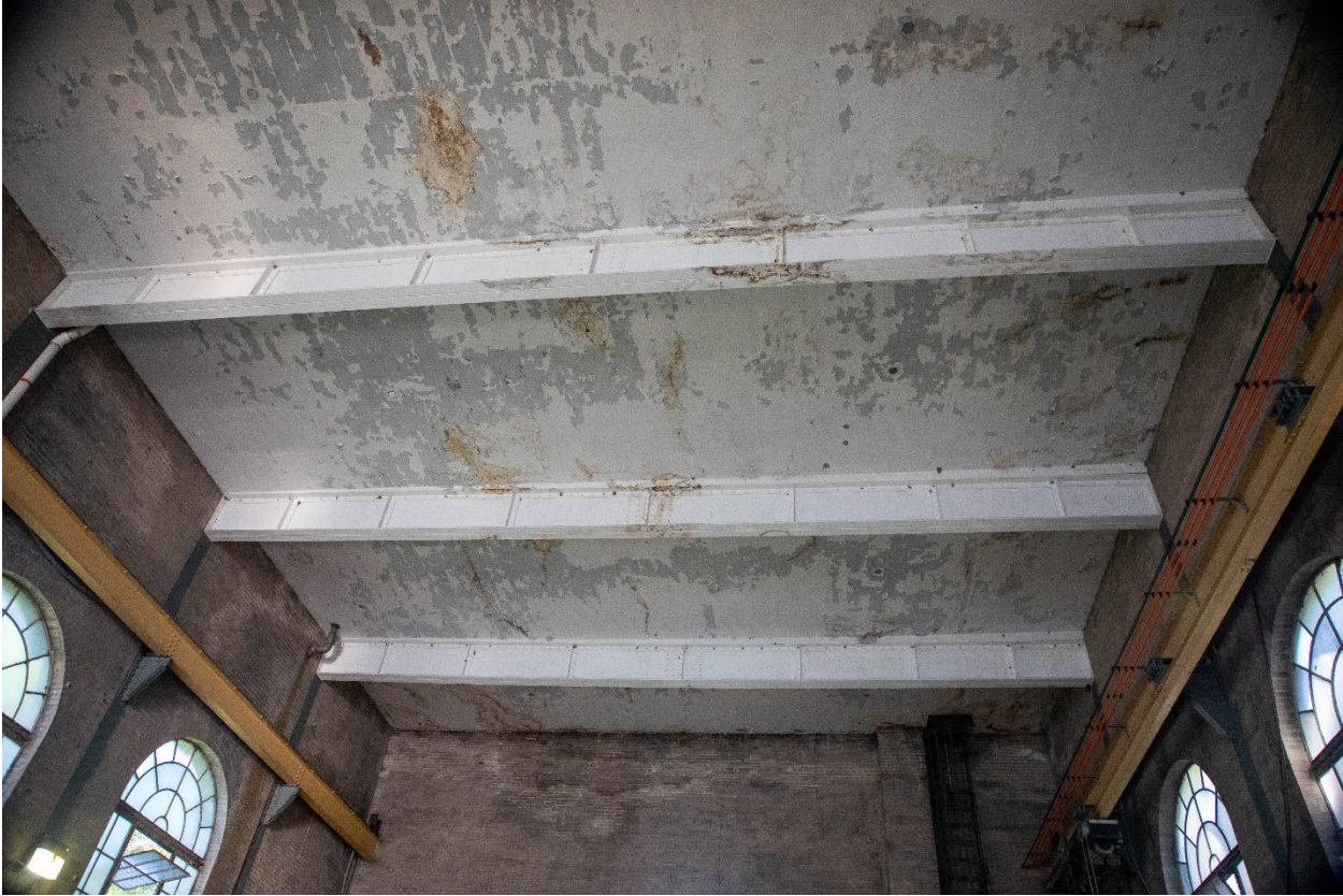
Water leaks through the roof structure.
